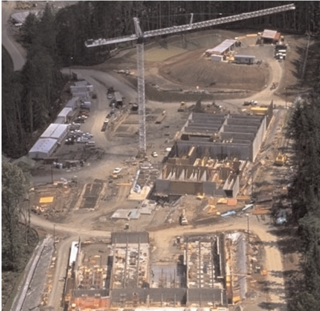
Tampa Bay Water's plant will be an ozone plant much like the Seattle Tolt facility.
